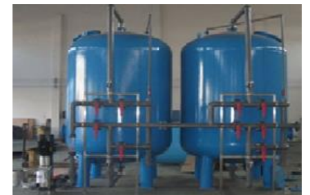
Rainwater Harvesting & Reuse System
