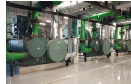
Hybrid Chiller Plants
