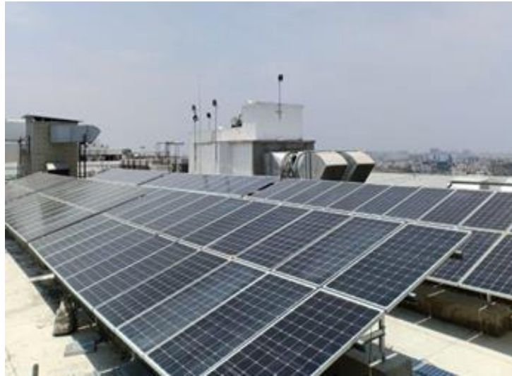
Solar Panel @ Rooftop
