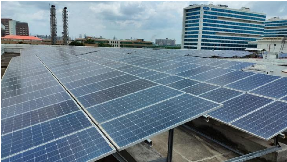
Solar Panel @ Rooftop
