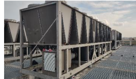
Air Cooled Chiller
