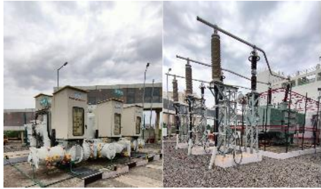
110 kV GIS & Transformer
