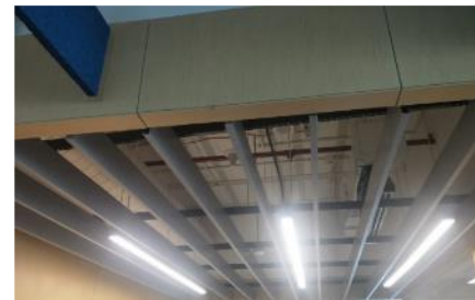
LED Lighting System
