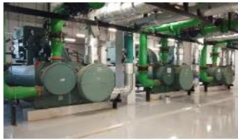
Water Cooled Chiller
